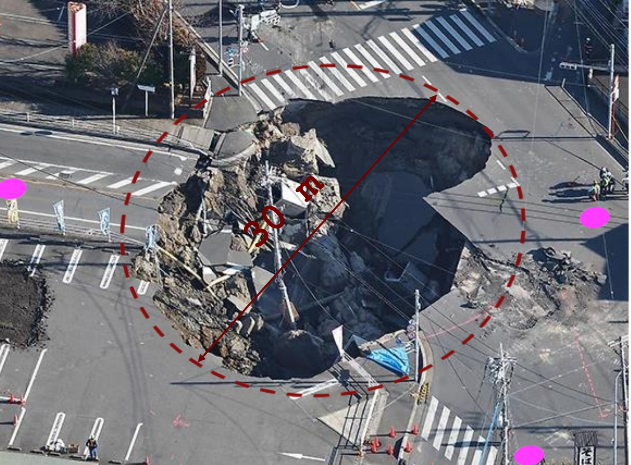
Yashio sinkhole incident (Saitama, Japan) *
